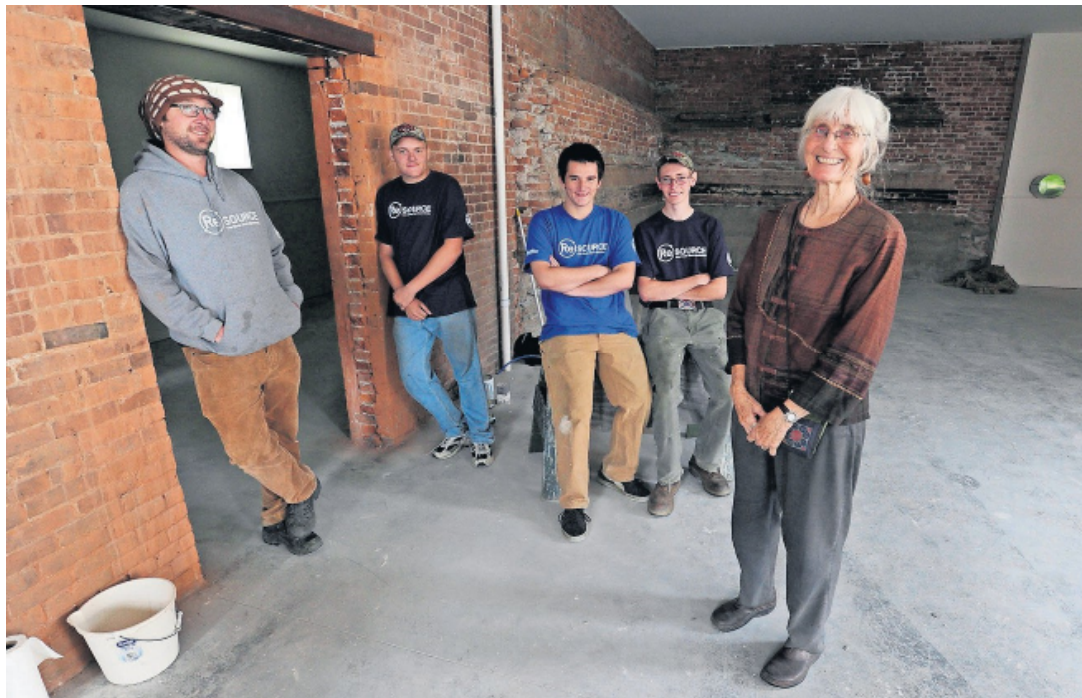
The Rise Up Bakery in Barre receives a big infusion of labor from the ReSource Youth Build program and new funding with a federal grant as they renovate the historic bakery. From left are Youth Build Manager Jesse Greig, students Michael Deedham, Matt Bailey and Hunter Larrabee, and project coordinator Carolyn Shapiro. JEB WALLACE-BRODEUR / STAFF PHOTO
